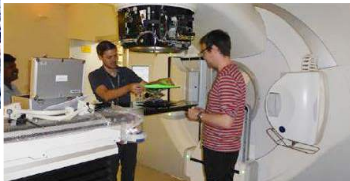
LTHT Medical Physics staff installing LINAC machines in the Sir Anthony Mamo Oncology Centre (SAMOC) in Malta
